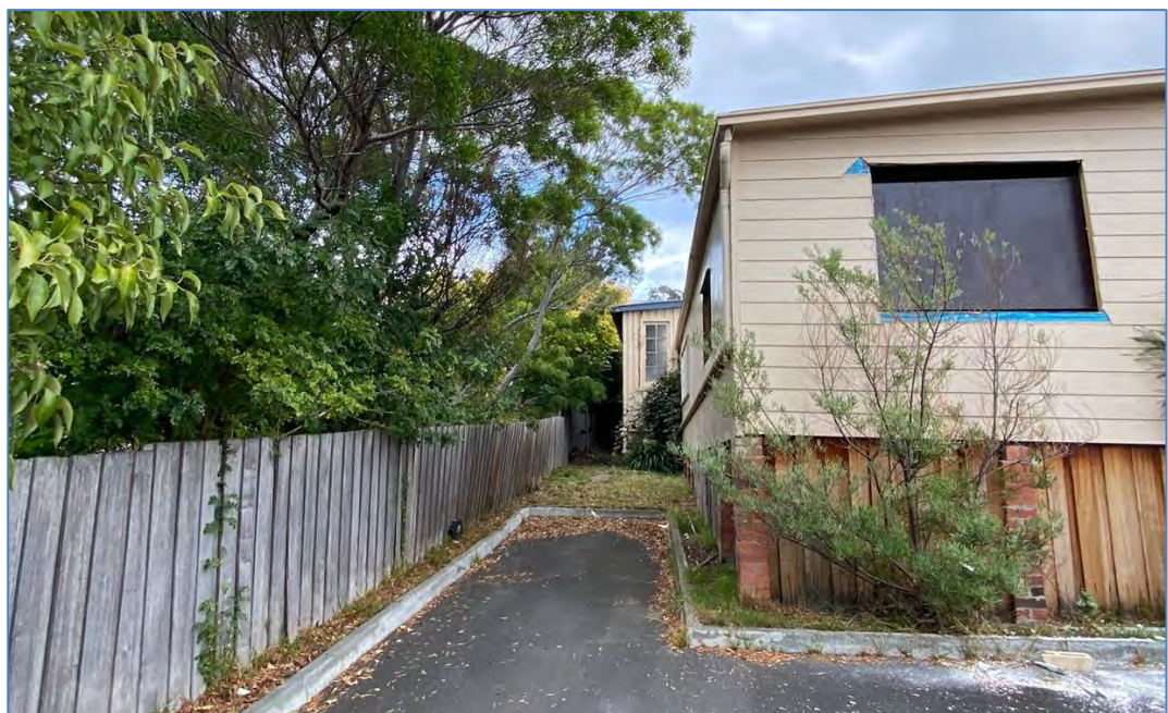
Figure 8 - Side boundary with buildings to be demolished and location of new deck.
